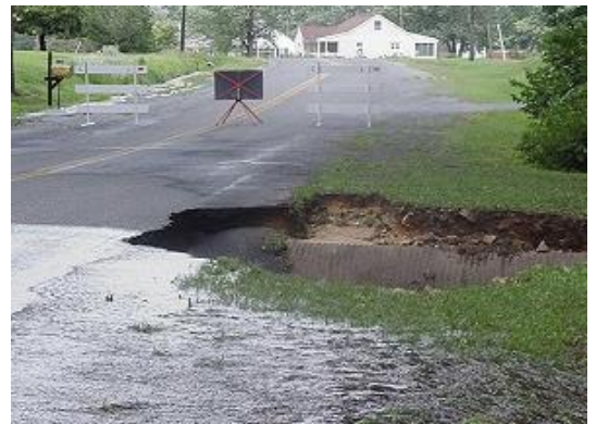
Figure 4-9: Road Closure Due to Flooding
